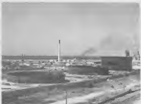
whole series of tanks that went up recently near the garage. Chicago Bridge, the contractors, chose to work on all six tanks simultaneously ter un serie di tanki cu a wòrdè erigí ricientemente cerca di garage. Chicago Bridge, e contratistanan, a traha ariba tur seis tanki na mes
